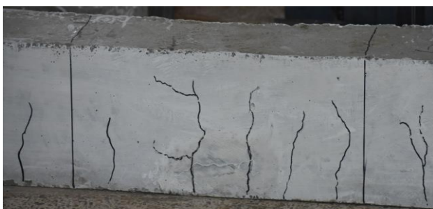
Figure.3: CB Crack pattern
