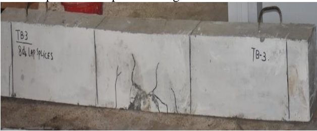
Figure.6: The TB3 crack patterns
