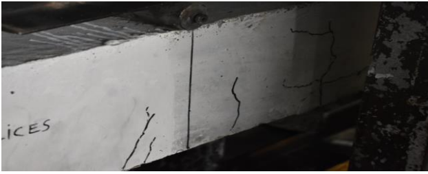
Figure.5: The TB2 crack patterns
