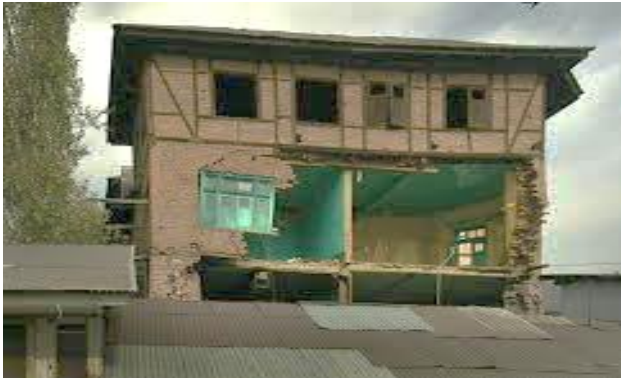
Figure 5: Unreinforced wall collapsed whereas the timber frame masonry section is still standing despite inertia
