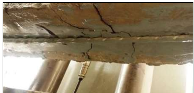
Figure 7: Debonding of GFRP rod shown on Photo of Beam B-5
