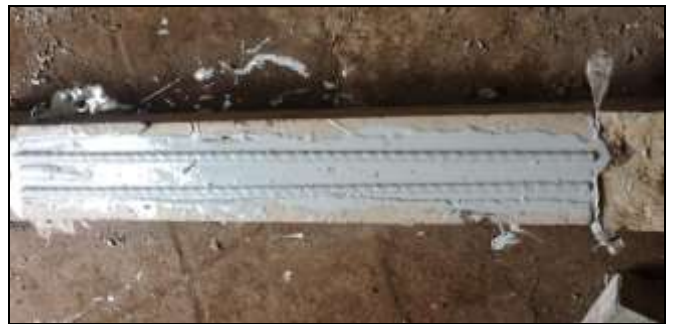
Figure 3: FRP rod inserted into epoxy resin at the bottom surface of the beam
