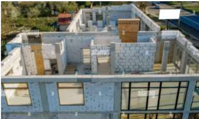
Figure 2: Building site of a house under construction made from white foam concrete blocks [9]
