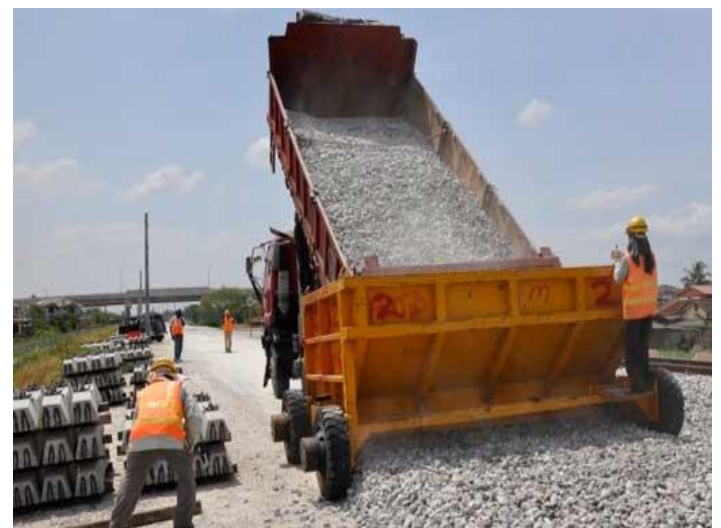
Figure 6: The track geometry is also more durable with a consistent ballast bed, while uneven ballast increases the danger of buckling.
