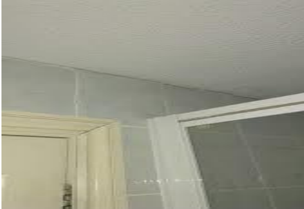
Figure 3: Horizontal cracks in the topmost story below slab level
