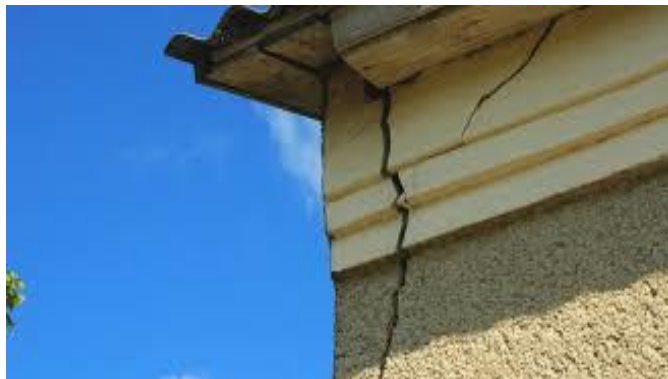
Figure 1: Cracks at ceiling level
