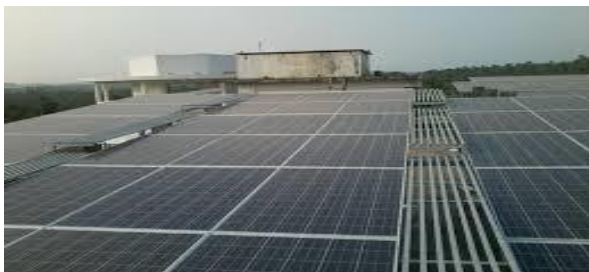
Figure 8: Rooftop solar was implemented on a public building
