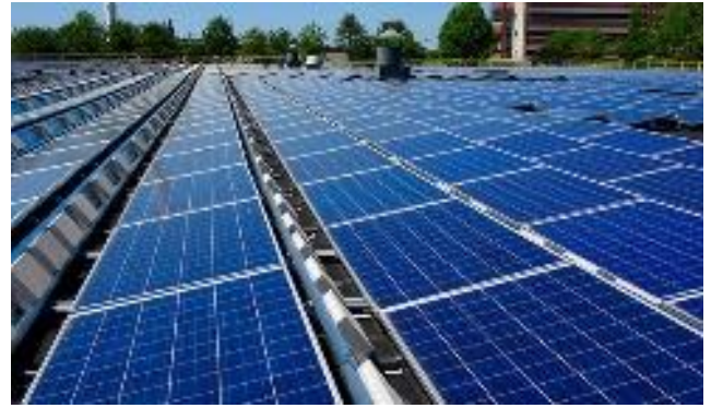
Figure 2: Solar Panel Array
