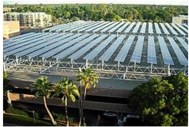
Figure 2: Solar Panel Array
