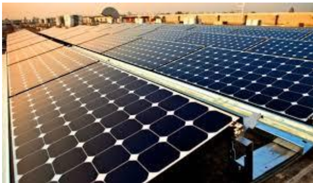
Figure 1: Solar panel field
